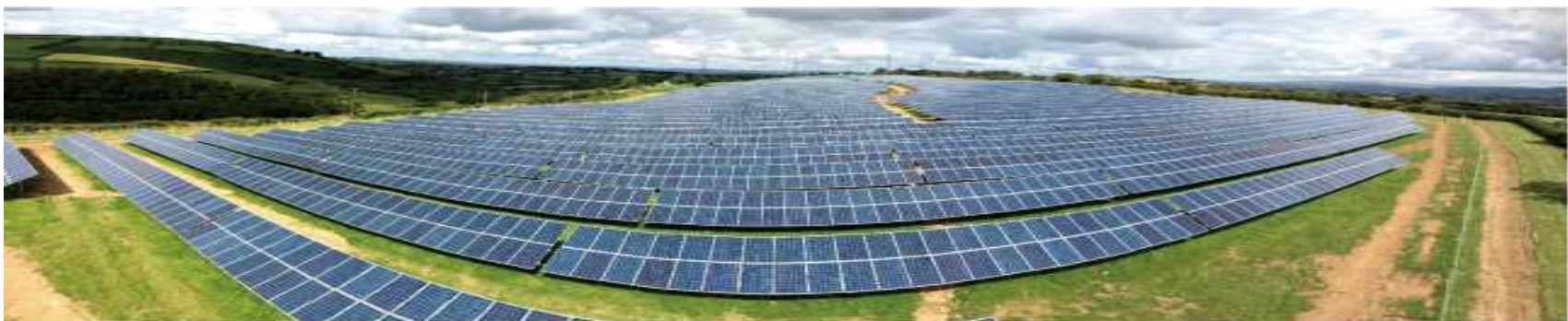
英国40MWRaventhorpe Farm地面光伏电站项目 40MWRaventhorpe Farm Ground PV Power Station, England
